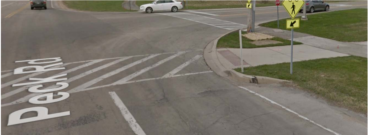
Figure 8 – Existing Southeast Curb Return Damage
